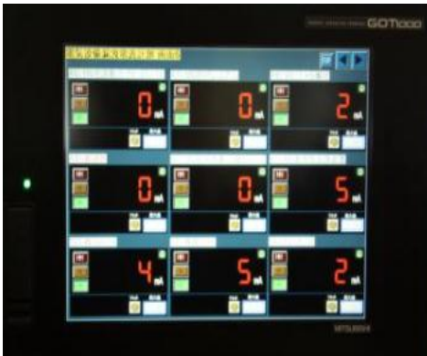
Continuous and Threshold Monitoring Display For Electrical Leakage
