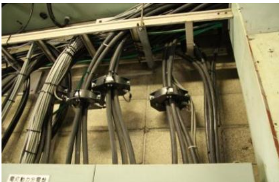
Electrical Leakage Detection Mounted At the Base Of the Panel Boards
